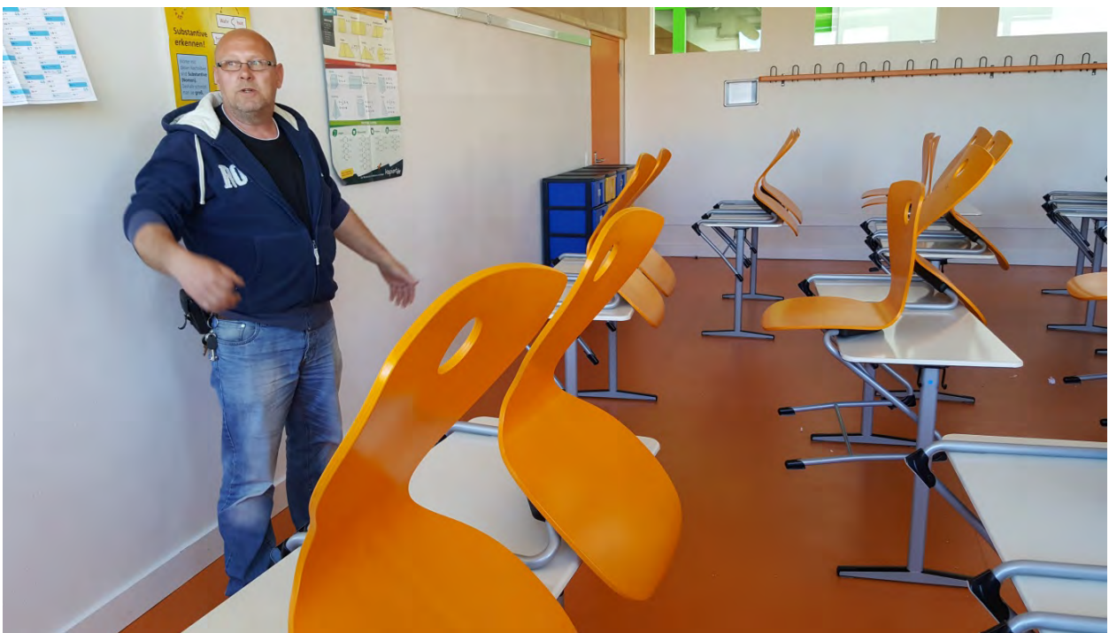
Facilities Manager Torsen Hillinger is extremely pleased with the ThermaSkirt heating system
