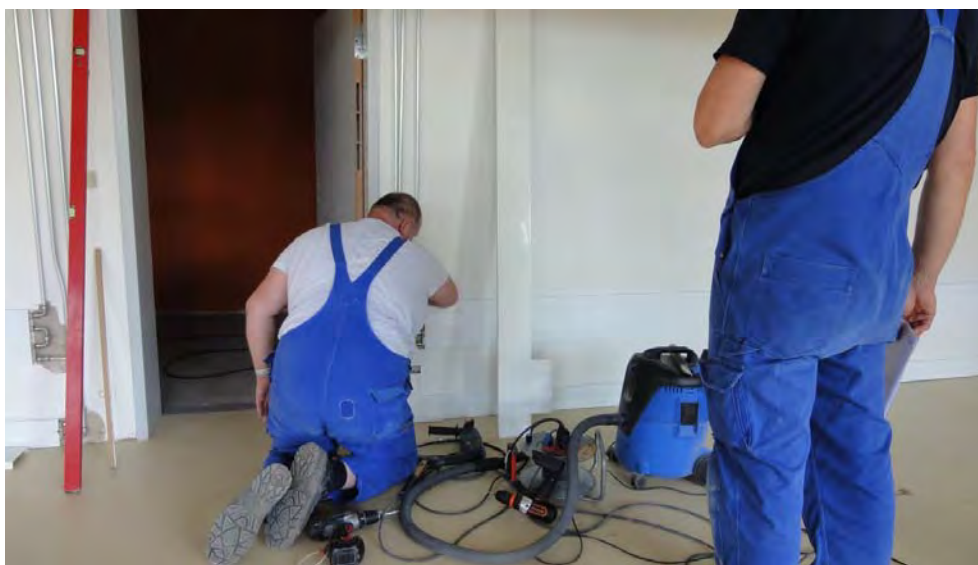
ThermaSkirt Germany designed, installed and commissioned all the ThermaSkirt systems
